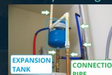
Expansion tank & pipes
