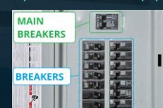
Electrical panel breakers
