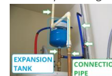
Expansion tank & pipes
