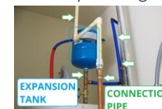
Expansion tank & pipes
